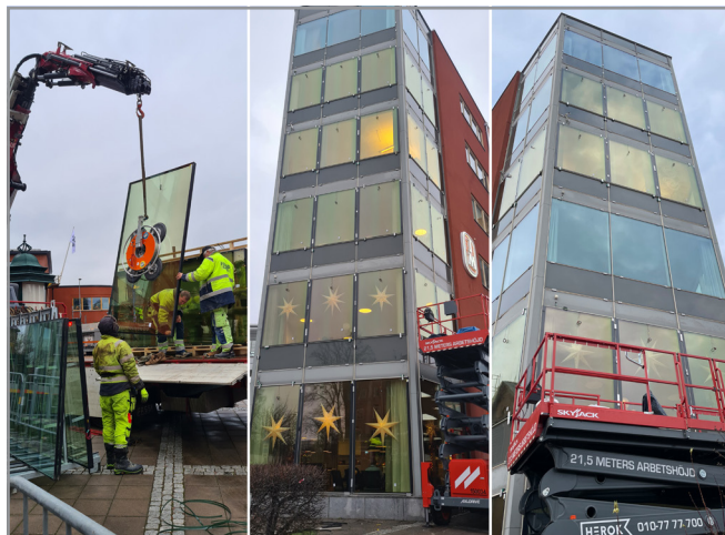
Installation of first insulating glass units with switchable electrochromic layers in December 2022 in Uppsala, Sweden
